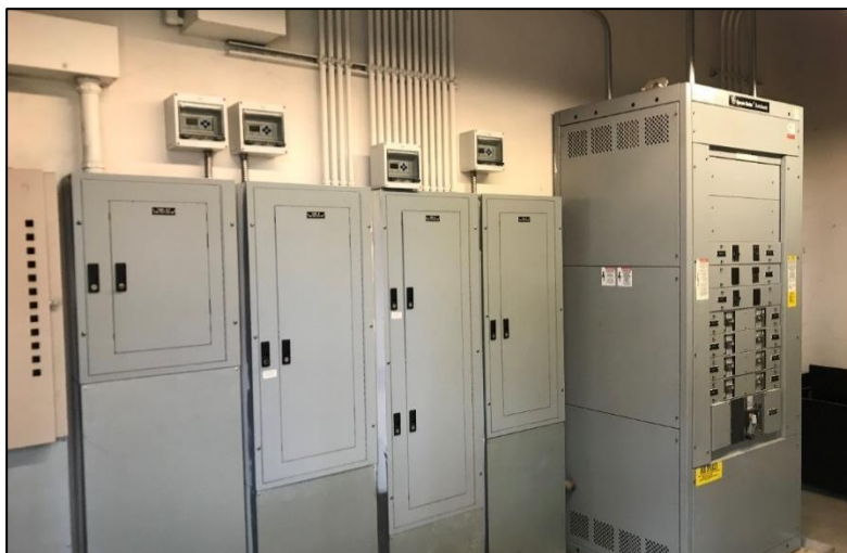
Figure 10: Autani Wireless Packaged Meters Connected to Electrical Panels
